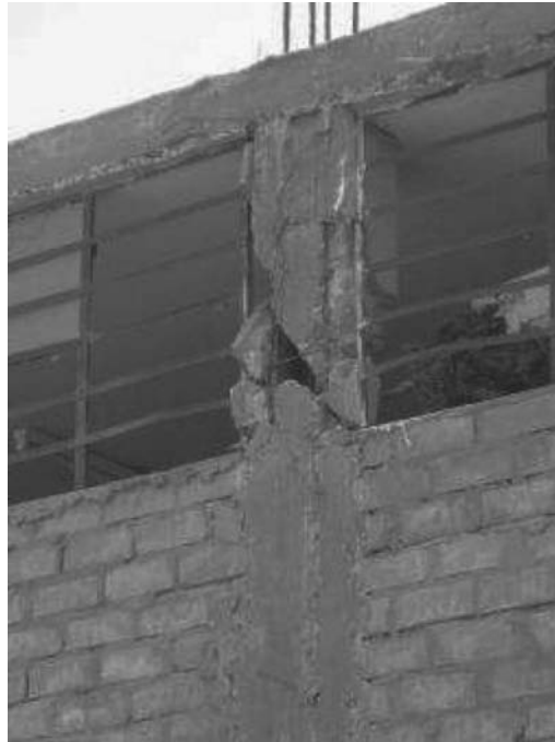
Figure 21.6 Damage to RC column (Pisco, Peru, 2007).
